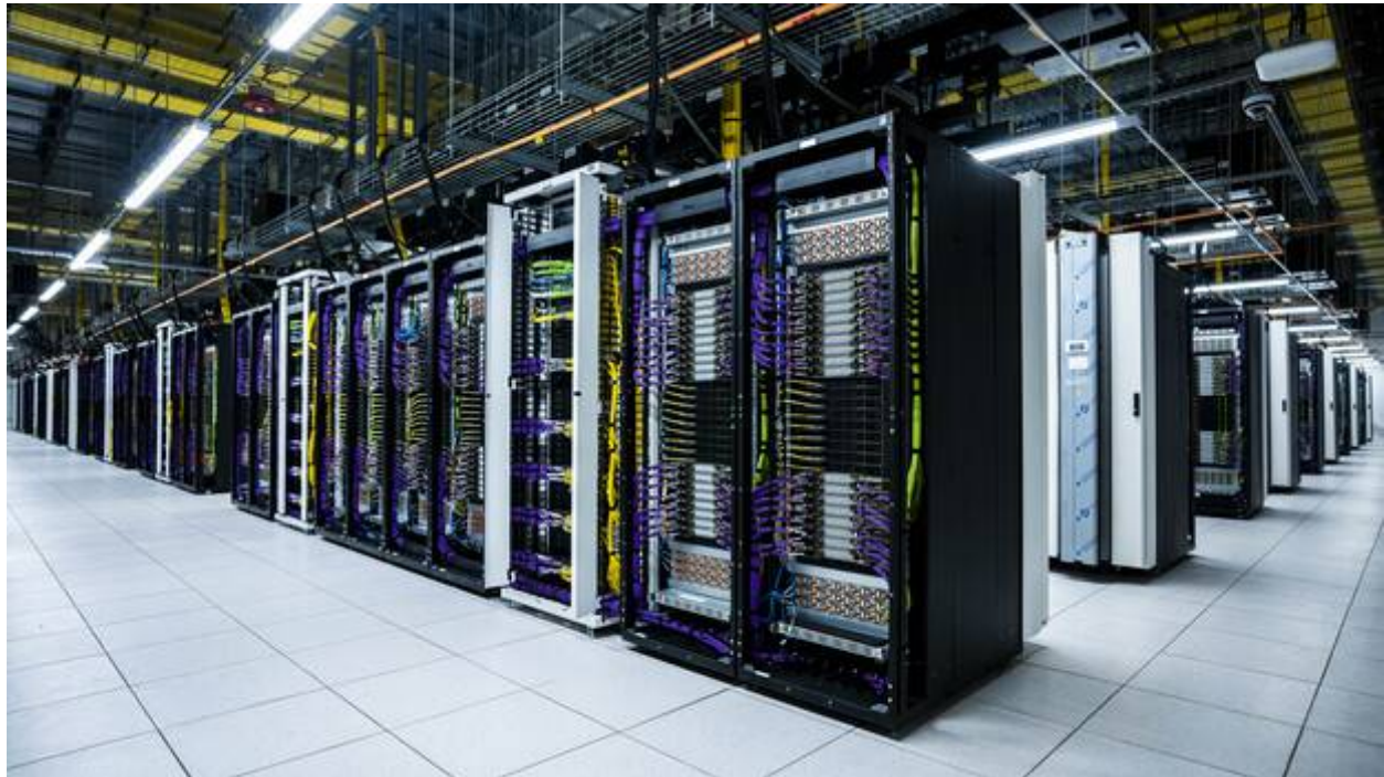
COLOSSUS II Facility in Memphis, Tennessee
